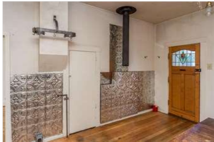
The pipe is from the huge propane cookstove they removed. Piping still there....If you look closely to the left you will see the oven plug in. Never used.
